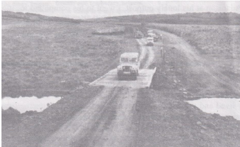
Small timber bridges built to open up tourist tracks for all season's use
